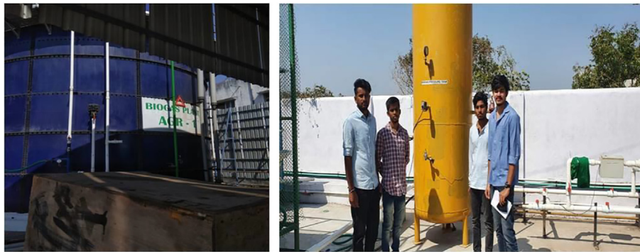
Fig. 9. (a) Anaerobic gas digester, (b) Bio gas pressure tank.
