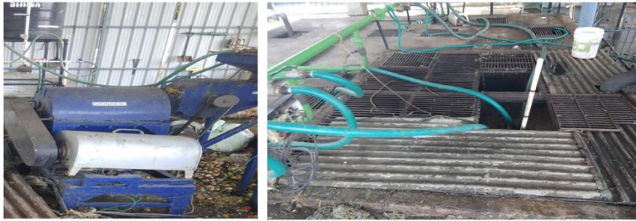
Fig. 8. (a) Grinder, (b) Sludge tanks hold organic vegetable waste.
